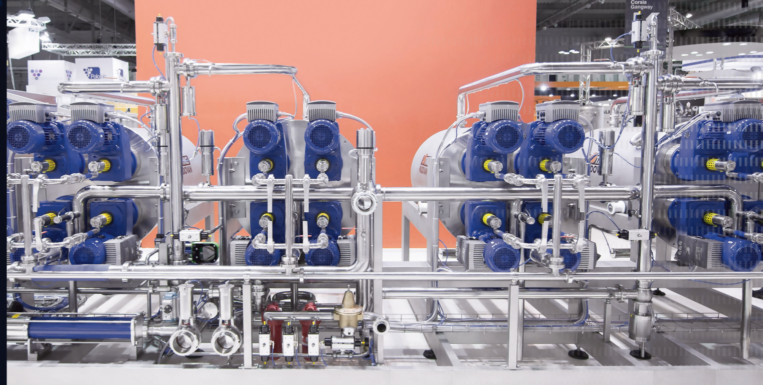
Novel filtration systems developed by TMCI Padovan help an Italian producer make highly authentic, full-flavored fortified wines. The innovative systems rely on distributed NORD drives for highly efficient operation.
